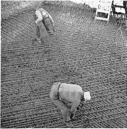
Placing reinforcing steel in tower foundation pits. A total of 35,000 pounds of steel was used for this purpose.
