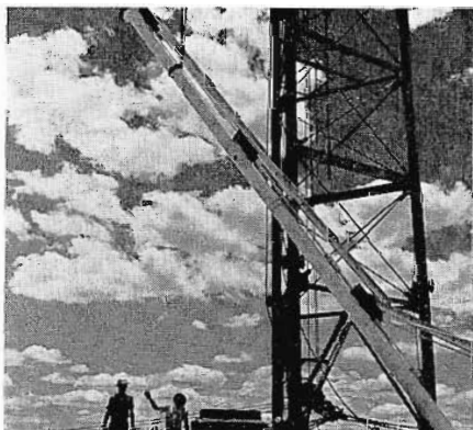
Rapid assembly of the tower structure is made possible by well-planned design and precise fabrication.
