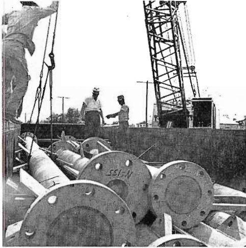
Solid rounds 30 feet long by 10 inches in diameter are hoisted from gondolas to waiting trucks.
