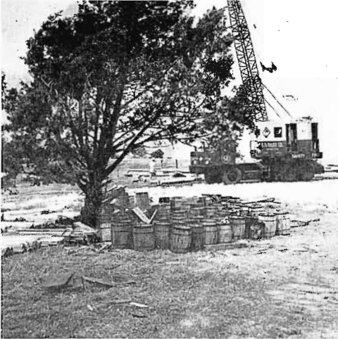
An old tree seems to offer shelter for some 50 kegs of bolts—"no need, they're galvanized!"
